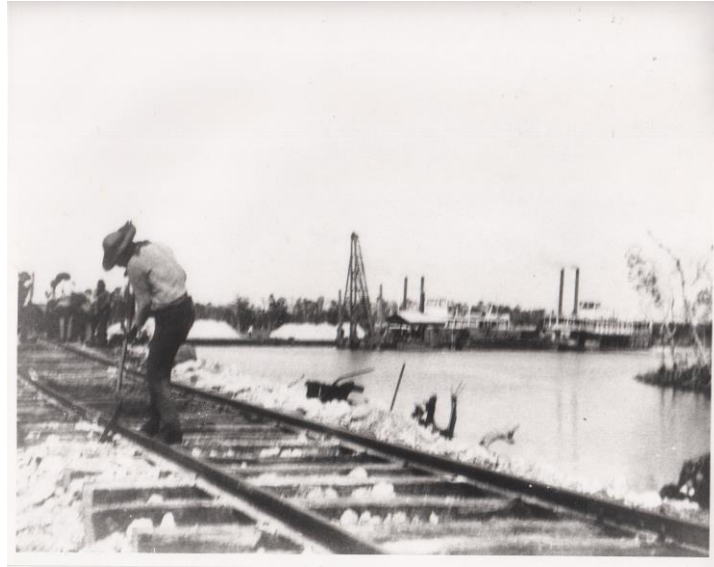
Black and white photograph of men working on a section of the Overseas Railway with steamships in the background.
