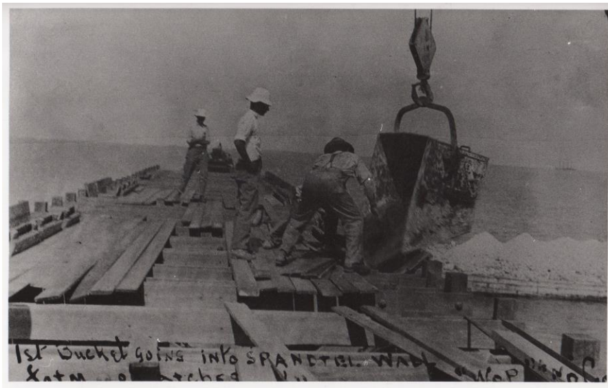
Black and white photograph of men working on a bridge belonging to the Overseas Railway. Possibly Long Key Bridge or Seven Mile Bridge.
