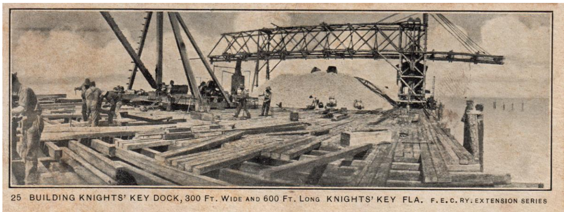
Building Knights' Key Dock, 300 feet Wide and 600 Feet Long, Knights' Key, Florida
